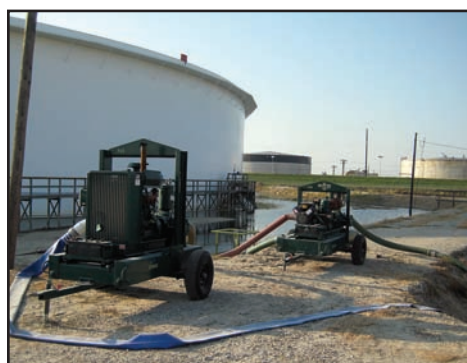
These pumps represent two of the 22 pumps from BakerCorp that a refinery staged around its plant in the event of high water during the hurricane season. The pumps went on rent on June 1 and will stay at the plant until Nov. 30.
